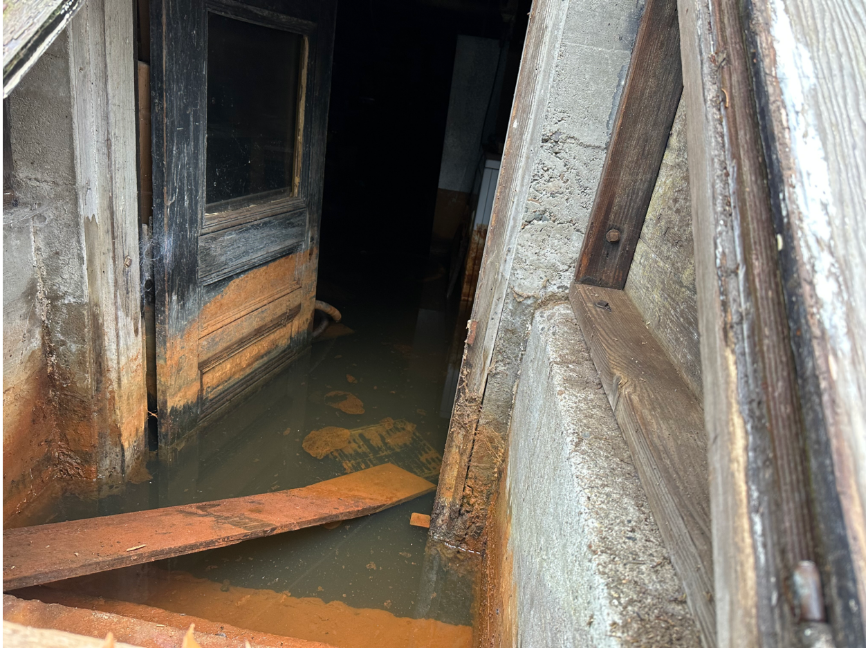
EXHIBIT C Photo of Flooding in House Basement
