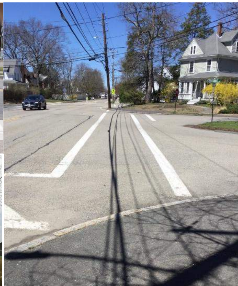
Lack of wheelchair ramps at Harris Avenue/Dedham Avenue
