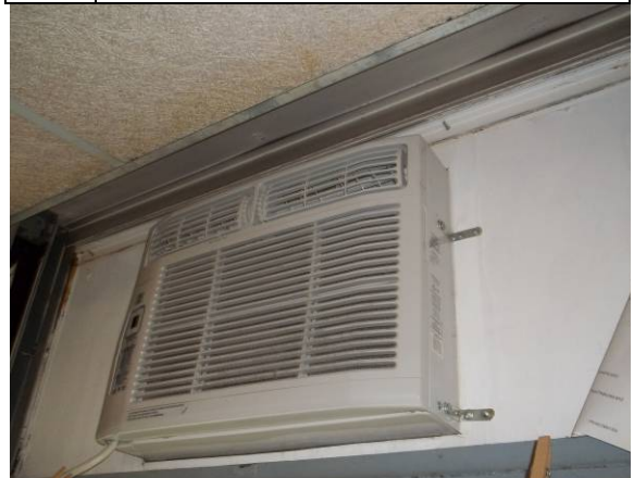
Photo #24: Window unit in classroom - 10,000 BTUH
