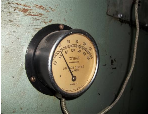
Photo #37: Supply temperature during onsite visit – providing outside air with no heating
