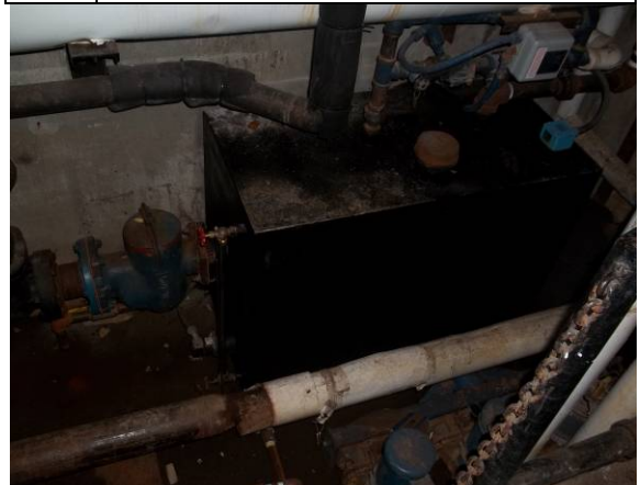
Photo #30: Condensate tank for low pressure steam system
