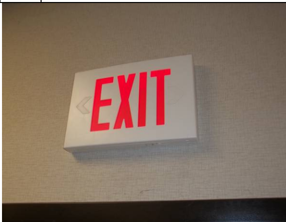
Photo #17: Exit lighting throughout building
