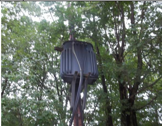
Photo #47: Pole mounted transformer
