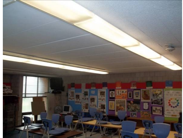
Photo #20: Classroom with T-8 lighting - uses wireless motion sensors
