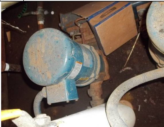
Photo #33: Condensate pumps – 0.5 hp
