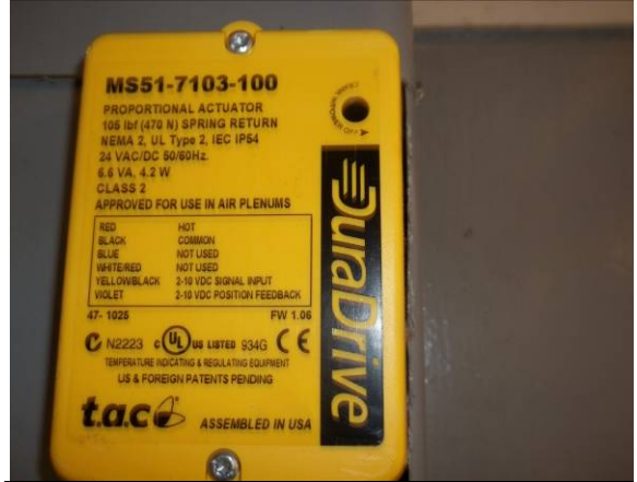
Photo #38: Actuators located on unit vents
