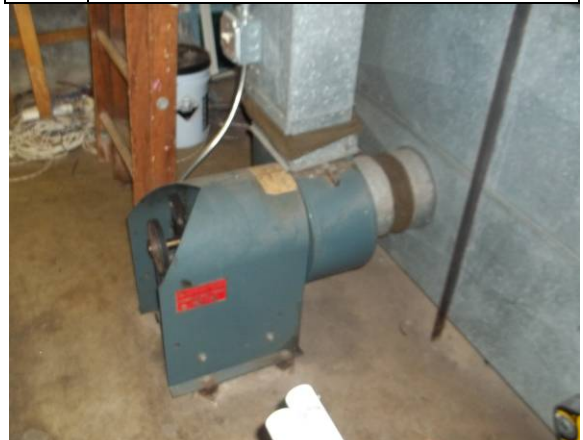
Photo #36: Return fan motor on air handling unit
