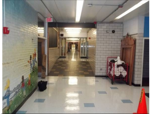
Photo #14: Ground floor main hallway – uses T-8 lighting
