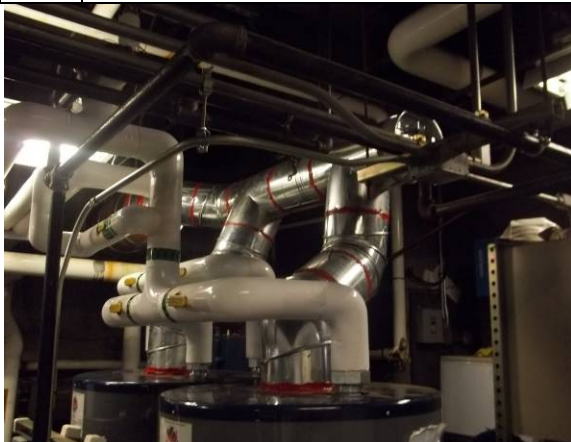
Photo #29: View of flue for domestic water heaters
