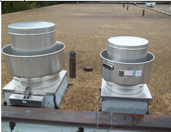
Photo #45: Kitchen exhaust fans
