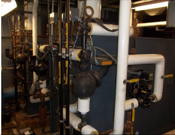
Photo #31: Low pressure steam boilers – operates in a lead lag format
