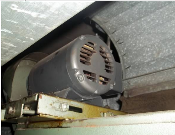
Photo #35: Supply fan motor on air handling unit
