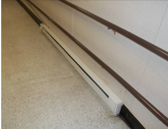
Photo #19: Electric baseboard heater in modular section
