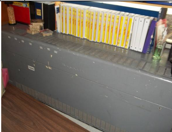
Photo #23: Unit ventilator in classroom
