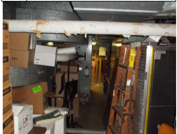
Photo #34: Air handling units with about 20-25% outside air - serves the gym and cafeteria
