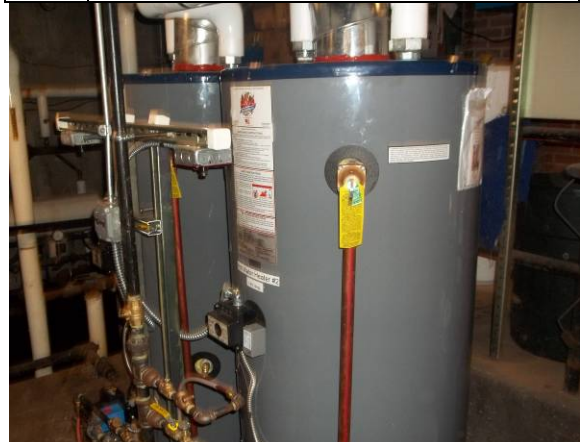
Photo #28: Domestic hot water heaters – installed in 2011, 1.5 GPH #2 oil
