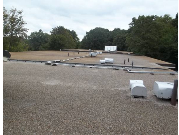
Photo #44: Roof of building – exhaust fans for bathrooms and kitchen areas
