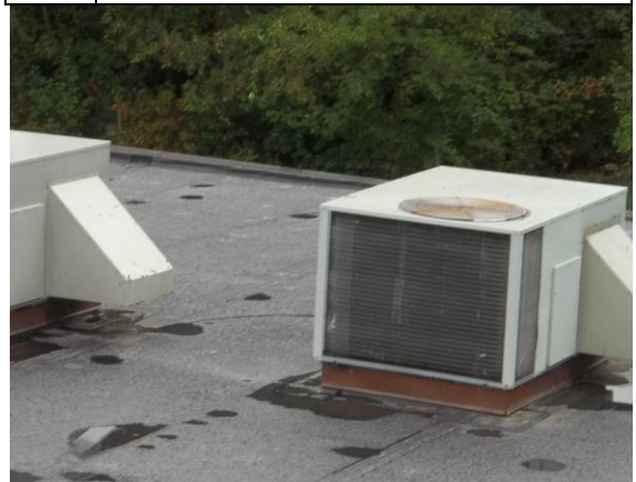
Photo #46: Packaged heat pump roof top units for modular section
