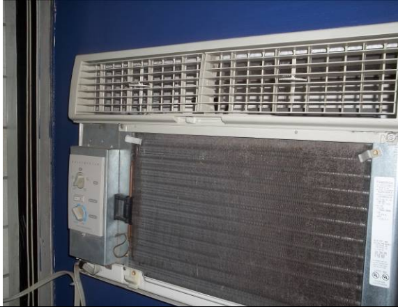
Photo #43: 28,000 BTUH window unit in classroom
