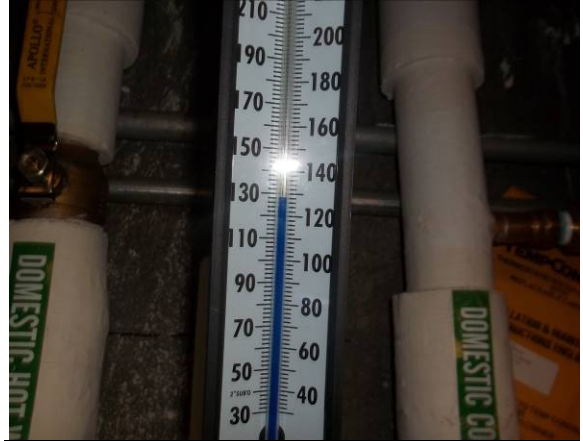
Photo #32: Domestic water temperature – measured at 140 degrees F during onsite visit
