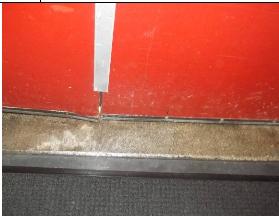
Photo #23: Internal view of door with air leakage issue – recommend weather stripping
