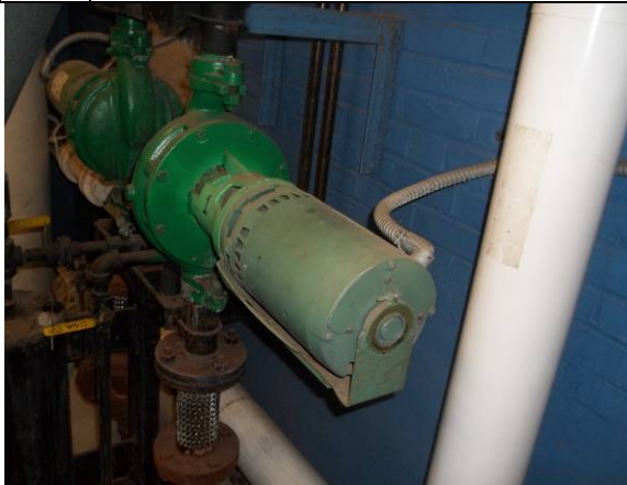
Photo #41: Condensate return pump
