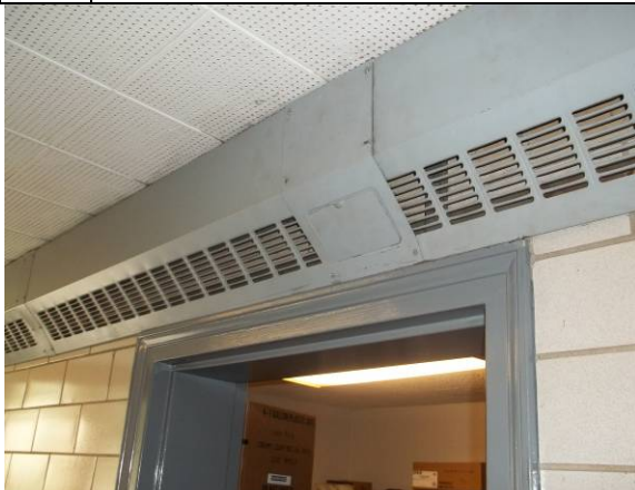
Photo #35: Heating for hallways – using steam from central boiler system
