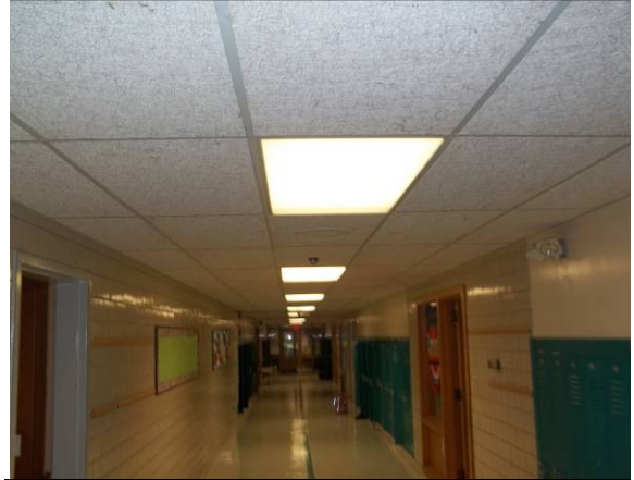
Photo #20: Hallway with T8 lighting
