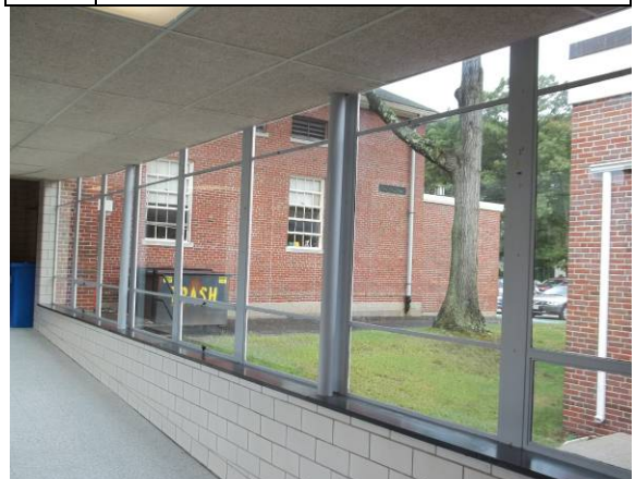
Photo #18: Internal view of hallway – recommend photo-sensors on these hallway lights
