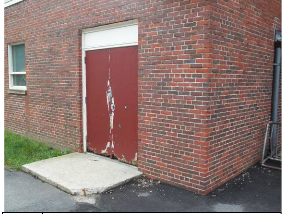
Photo #8: One of several entrance doors that should be replaced
