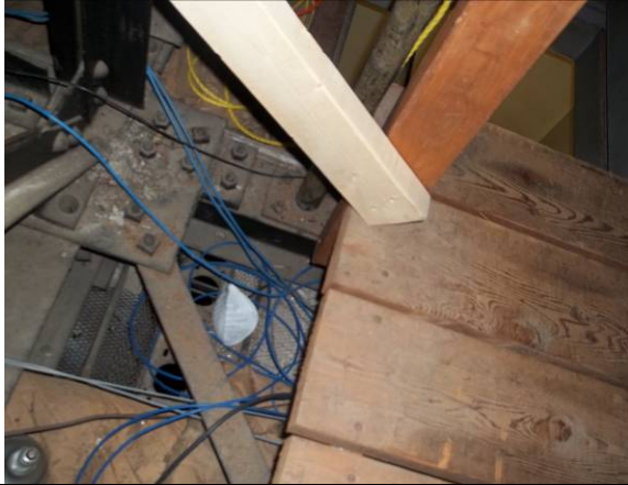
Photo #37: Another part of the attic –no insulation
