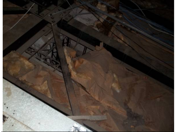
Photo #38: This part of the attic has less than 1 inch insulation
