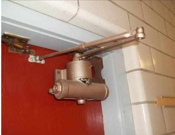
Photo #31: Hydraulic door closer is broken resulting in the door not closing properly
