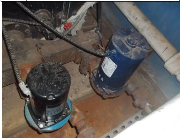
Photo #46: Additional condensate pumps located on return line - located in storage room
