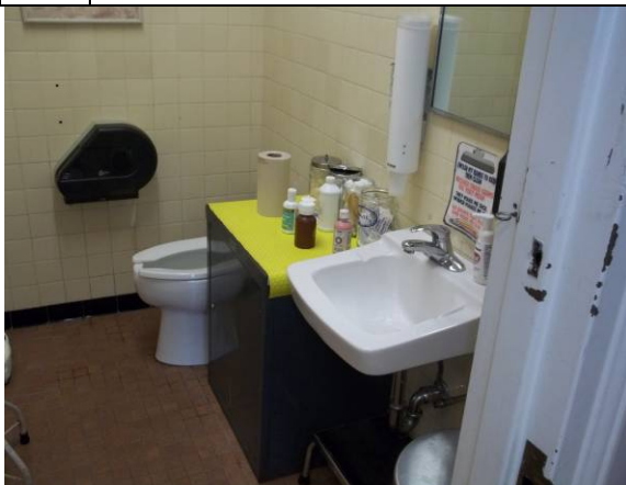
Photo #47: Toilet with 1.6 GPF toilets and 2.2 GPM faucet
