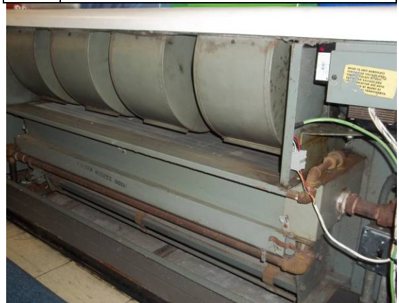
Photo #30: Internal system of unit vent.
