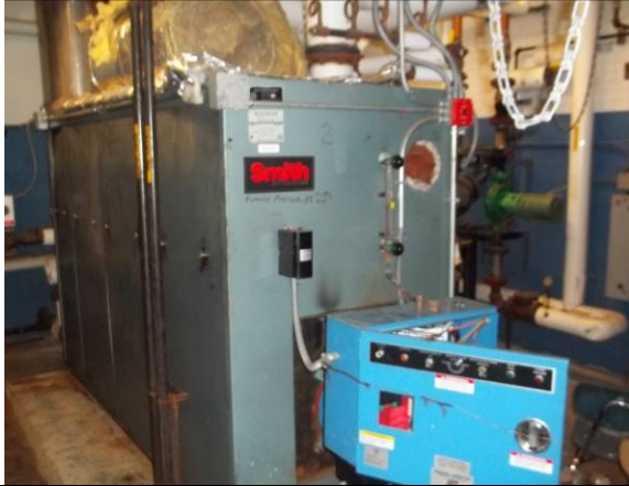
Photo #43: Second boiler
