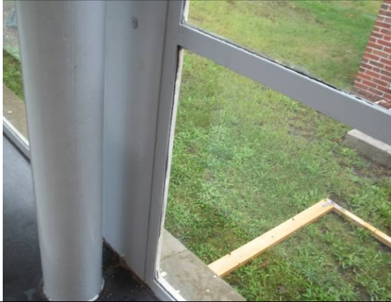
Photo #19: Single pane windows
