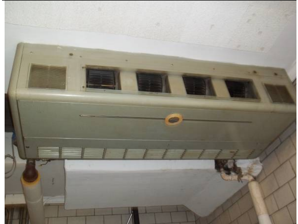
Photo #34: Fresh air unit for kitchen
