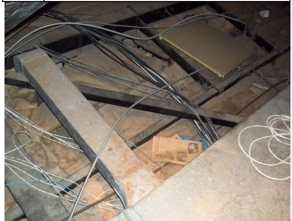
Photo #36: Attic – little or no insulation (this part of the attic has no insulation)
