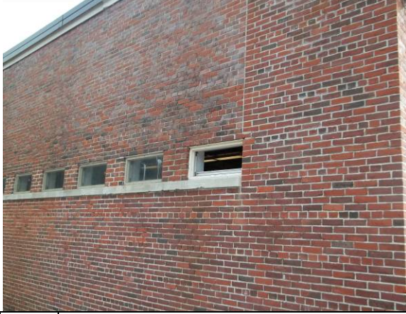
Photo #7: Gymnasium windows – in poor condition recommend replacement
