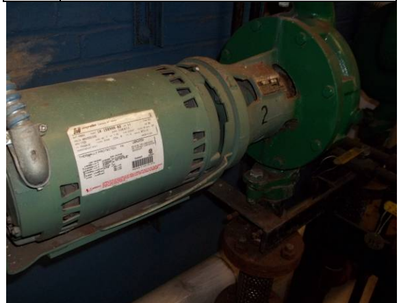
Photo #42: Additional view of condensate return pump
