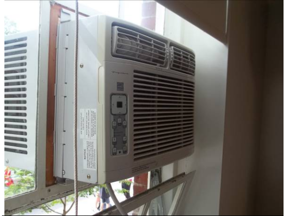
Photo #26: Window unit in classroom – 10,800 BTUH
