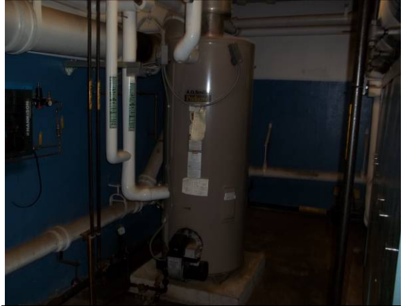
Photo #44: Domestic water heater – oil fired. 86 gallons - currently set at 140 degrees
