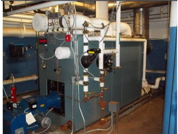
Photo #40: One of two #2 fuel oil-fired boilers used for heating - only one boiler needed for heating entire building
