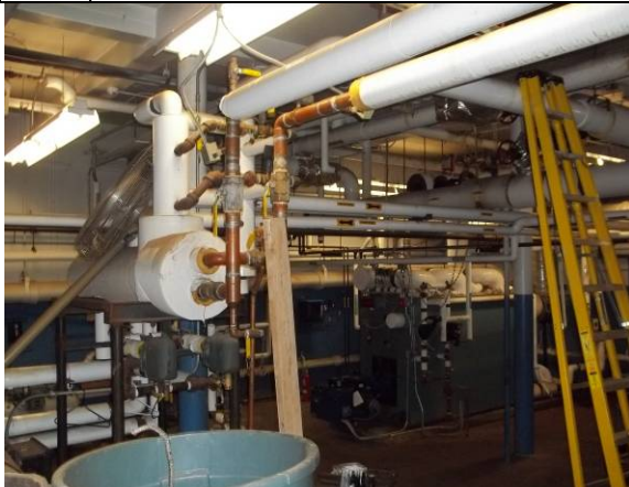
Photo #39: Boiler room
