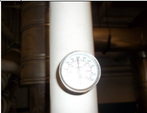
Photo #45: Temperature gage for domestic water – 140 degrees F
