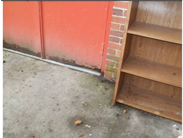
Photo #10: Another entrance door that should be replaced with a new door
