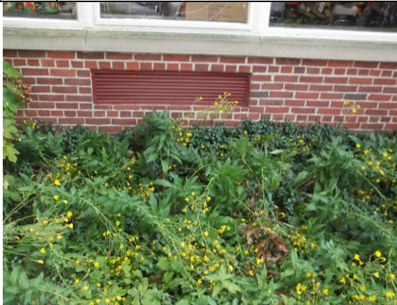
Photo #15: Unit vent – external grill (issues with air drafts through grill)
