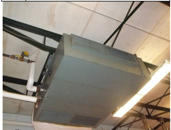
Photo #22: Air handling unit for gymnasium – can be heated with steam from central system
