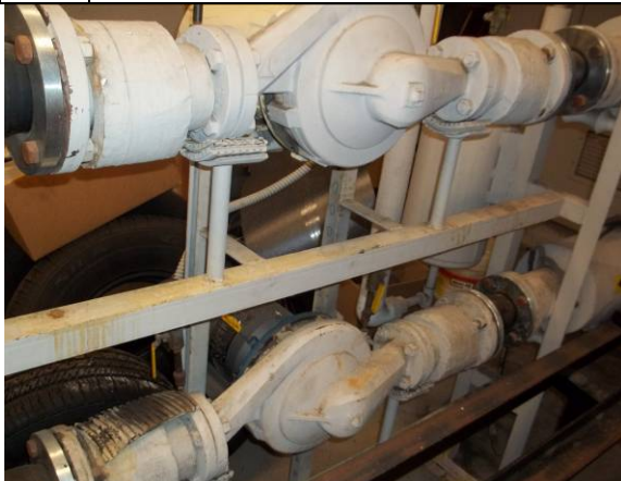
Photo #39: Hot water circulation pumps – 5hp, recommend VFD
