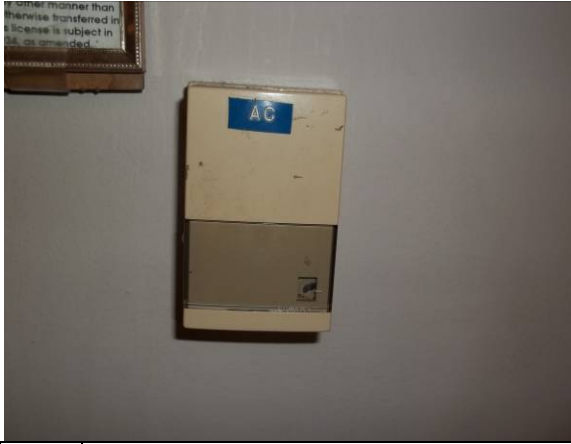
Photo #31: Cooling control
