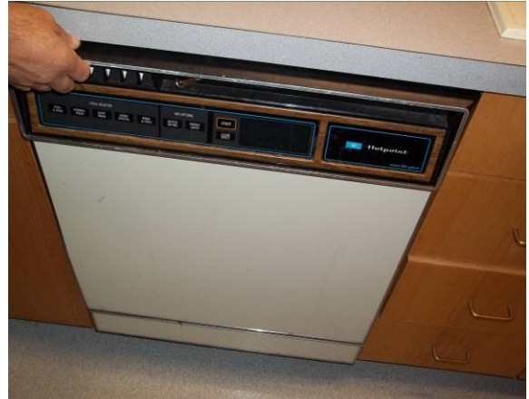
Photo #20: Dishwasher in kitchen in police department – recommend new dishwasher
