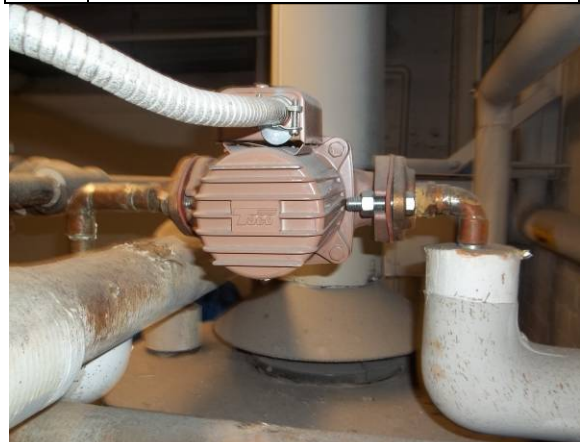
Photo #28: Domestic water circulation pump
