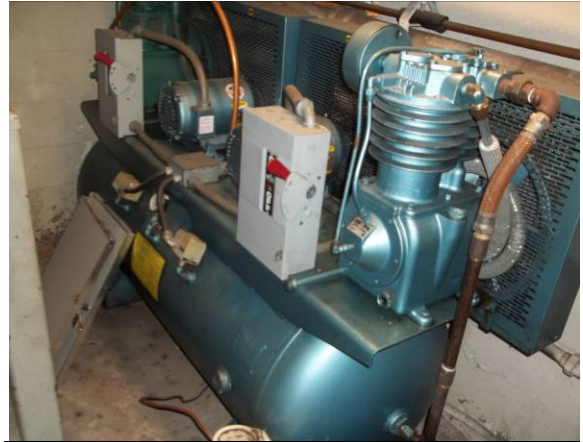
Photo #38: Compressor for pneumatic control system
