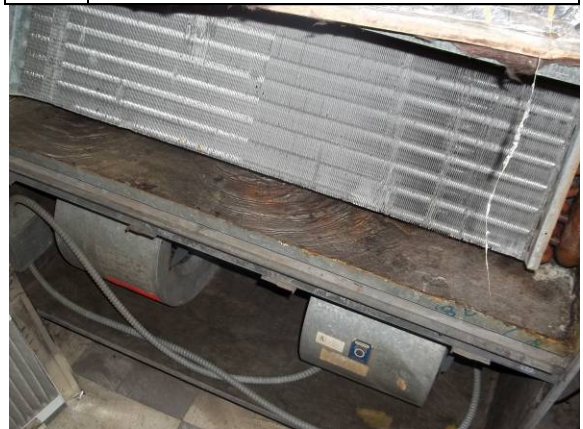
Photo #42: Inside of air handling unit. Has two 1/5 hp blower motors. Note standing water below the evaporator coil
