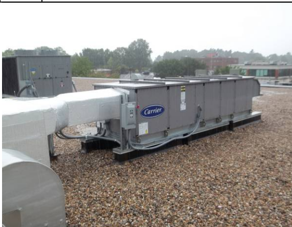
Photo #35: Make-up air unit
