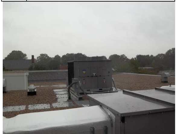
Photo #36: Chiller for building
