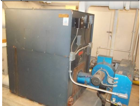
Photo #40: Boiler (1703 MBH) for hot water heating
