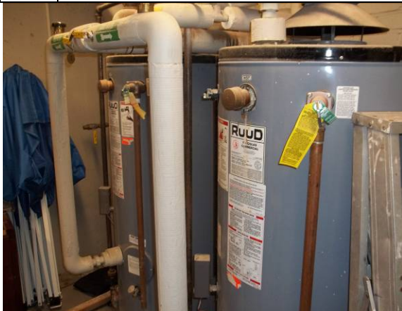
Photo #27: Domestic water heaters for entire building
