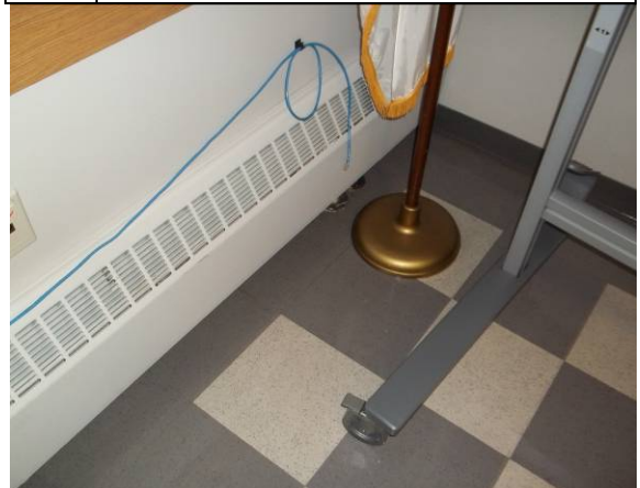
Photo #34: Hot water based radiator
