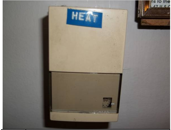
Photo #32: Heating control
