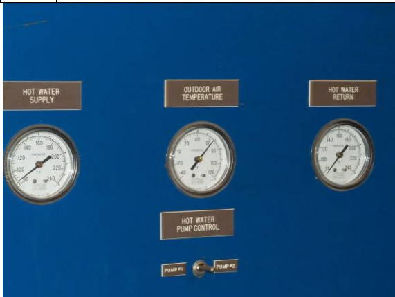
Photo #41: Hot water heating temperature gages
