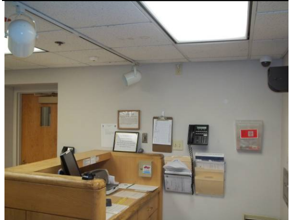
Photo #16: Booking room – recommend installing motion sensors
