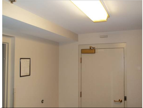
Photo #14: Lighting in hallway in police department
