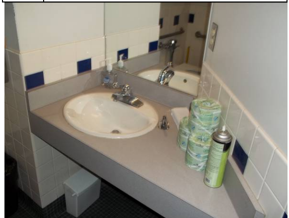
Photo #12: Restroom – have 2.2 gm faucets, 1.6 gpf toilets and timers on lights
