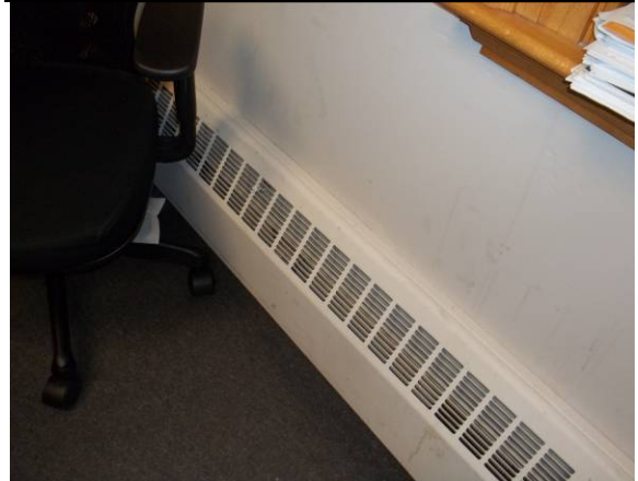
Photo #10: Hot water radiator used in both police and fire departments
