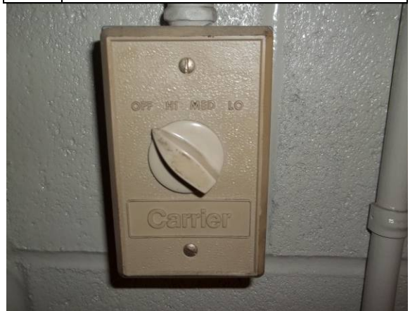
Photo #30: Control for blower in air handling unit
