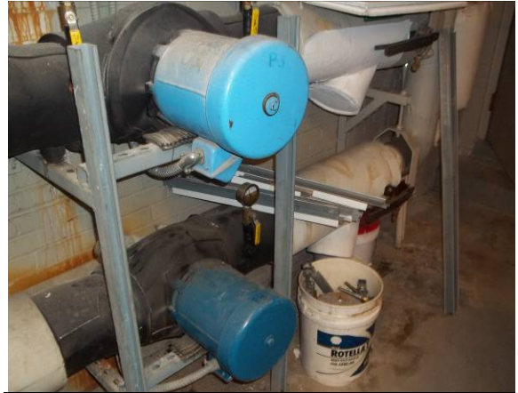
Photo #26: Chilled water circulation pumps – 5hp
