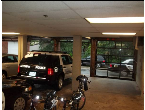
Photo #18: Garage with T-8 lighting – recommend removing some lights
