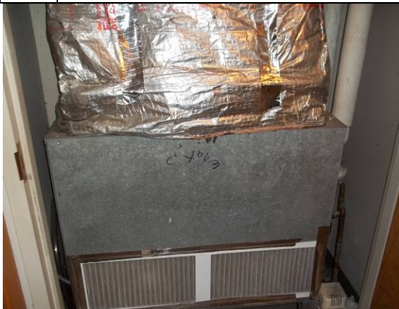
Photo #29: Air handling unit – cooling only
