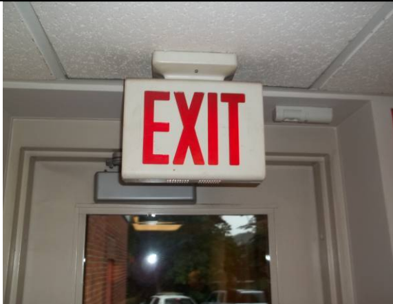
Photo #15: LED exit lighting
